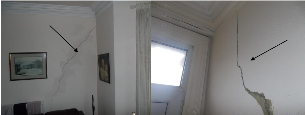
Cracking to the right-hand wall in the front lounge
