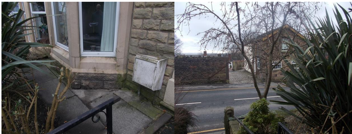
Front elevation and bay window. NB. The gas meter box is approximately in line with where the cracking is internally
